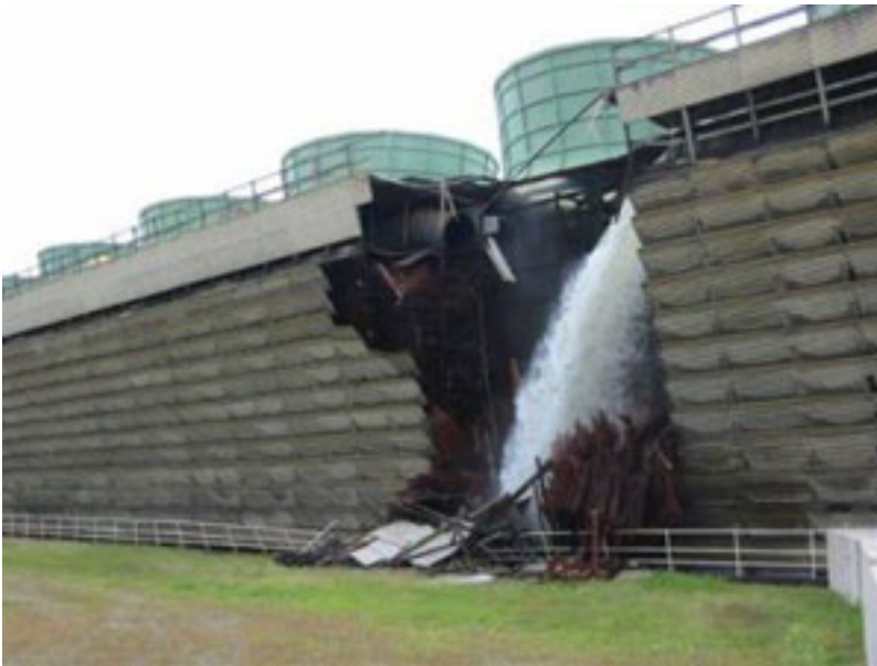
Cooling tower collapse, Vermont Yankee nuclear plant. Photo: Safe & Green Campaign
